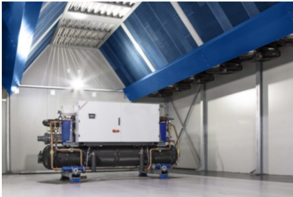
Example of water condensed unit inside Hyper Lab
